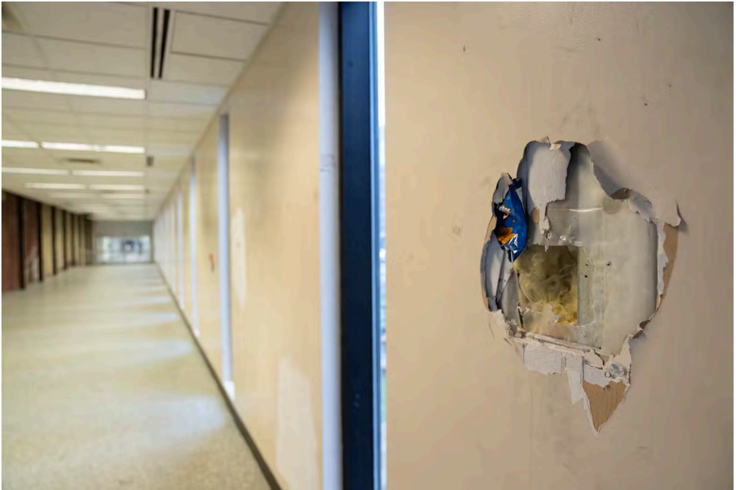
A hole in the wall of a downtown St. Paul skyway sits in disrepair in late 2023. City officials said administrative fines could be used to enforce building maintenance laws. (Alex Kormann)
